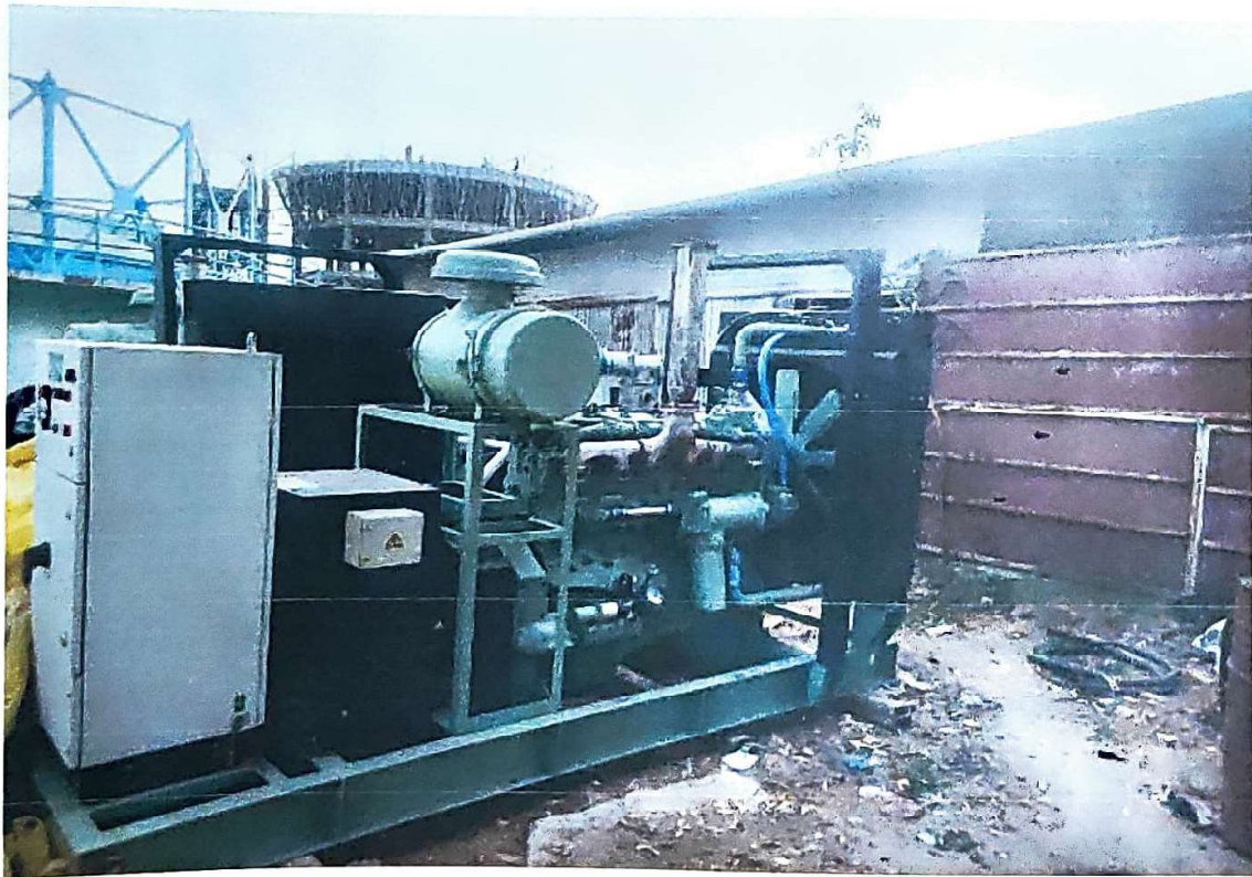
Gas Engine for Power generation
