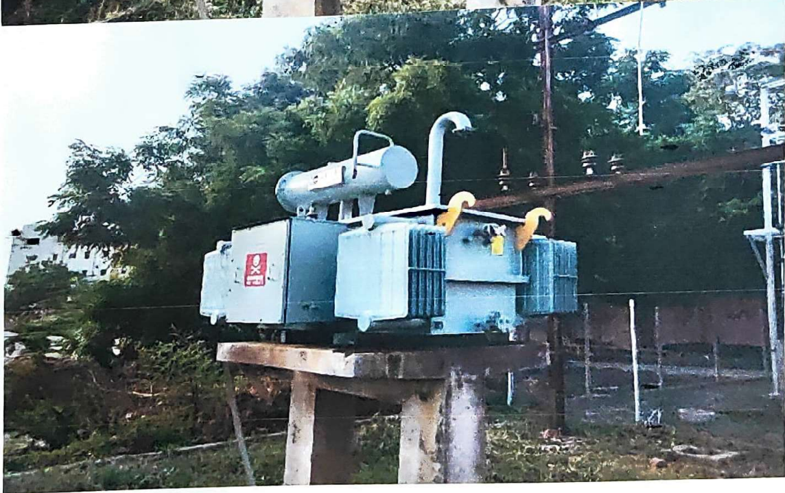
500 KVA Transformer Erected and Commissioned
