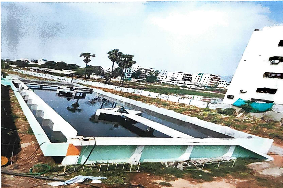
PRE AERATION TANK& DNT TANK
