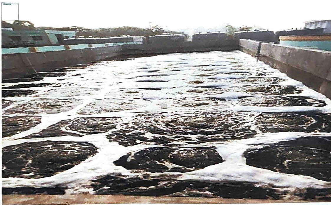
ADDITIONAL AERATION TANK
