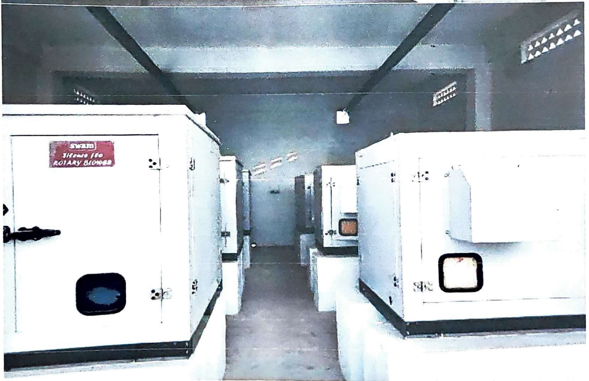
AIR BLOWER ROOM at RL Nagar
