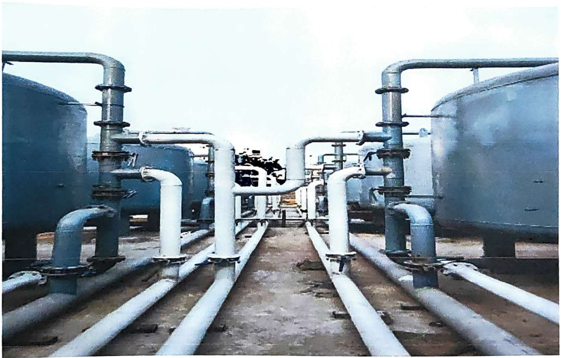
Pressure Sand Filter at RL Nagar for Tertiary treatment Completed
